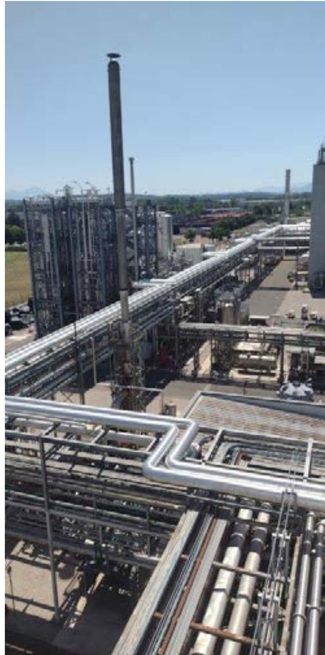
Trigeneration plant at the Patrica plant.
