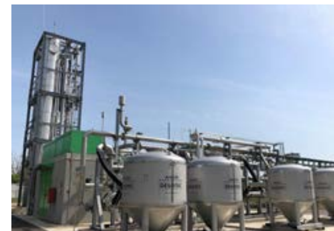
Biomethane production plant at the Bottrighe plant.
