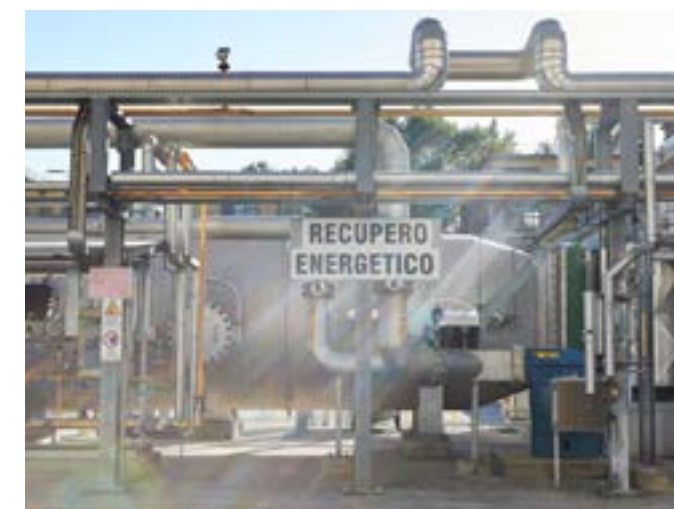
Energy Combustor at the Terni plant.
